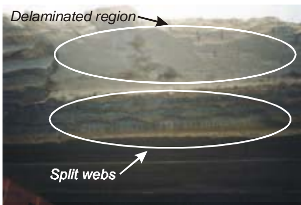
Figure 4. Delaminated section of hollowcore topping
