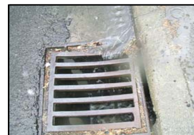
Fig 21: Drain on Ilam Rd that leads to Okeover via a 500 Ø culvert
