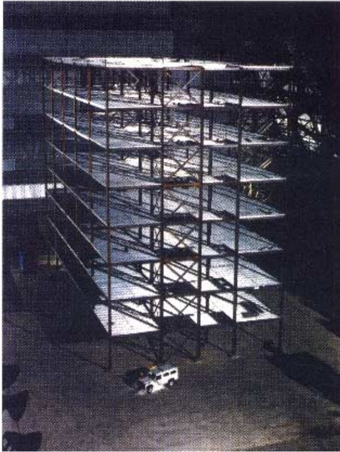
Figure 2.26 General view of the structural frame at the Cardington test (British Steel, 1999)
