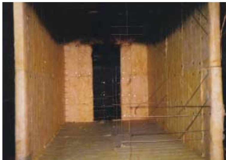
Figure 2.2 The Intermediate Service Board used to line the Interior of the two-compartment structure.
