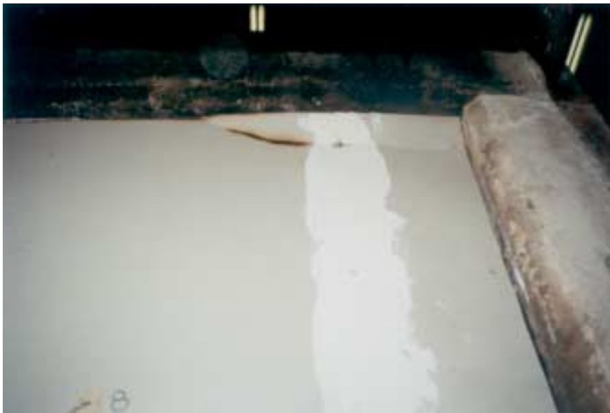
Figure 7-4: "Push-out" of the unexposed gypsum lining.
