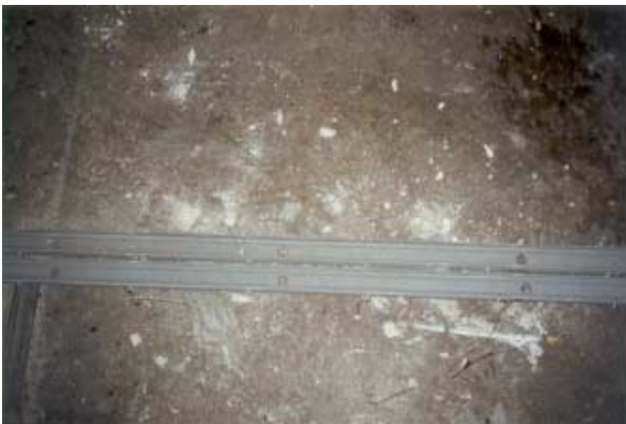
Figure 7-3: Relatively unaltered studs after furnace test FP2882.
